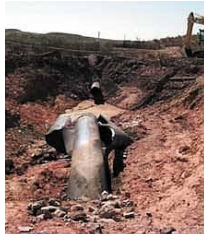
Carlsbad Natural Gas pipeline explosion, New Mexico, 19 Aug 2000
